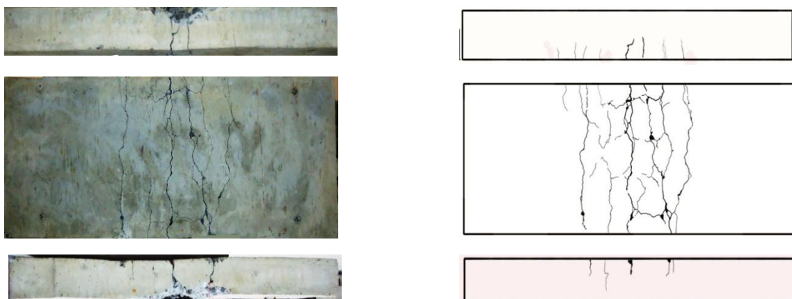
Fig 14: Cracks Pattern of Control Slab (A)
